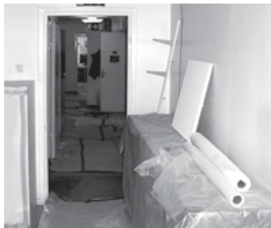
Work in progress - everything covered and sealed while the new pipes and services are put in all around us
