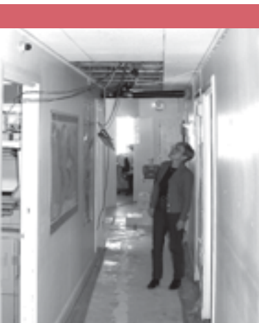
Cecilia Biriell checking part of the major building work which took place at the UMC offices
